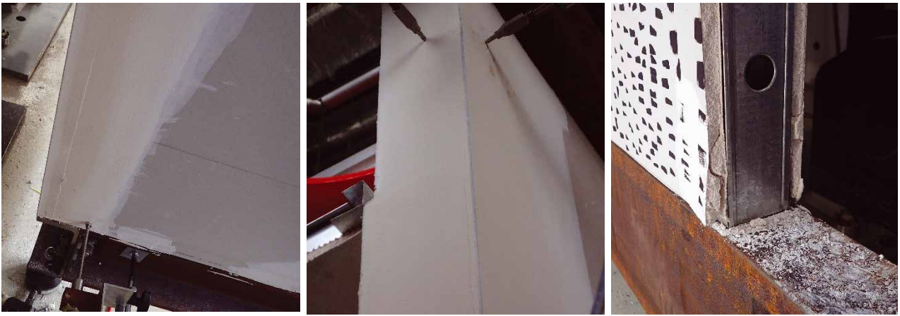
■ PHOTOS 3,4 & 5 – R2 L/360 ( \pm 5.40\text{MM} ) EXTERNAL CORNER, NIB WALL END, DOOR OPENING BASE DAMAGE
