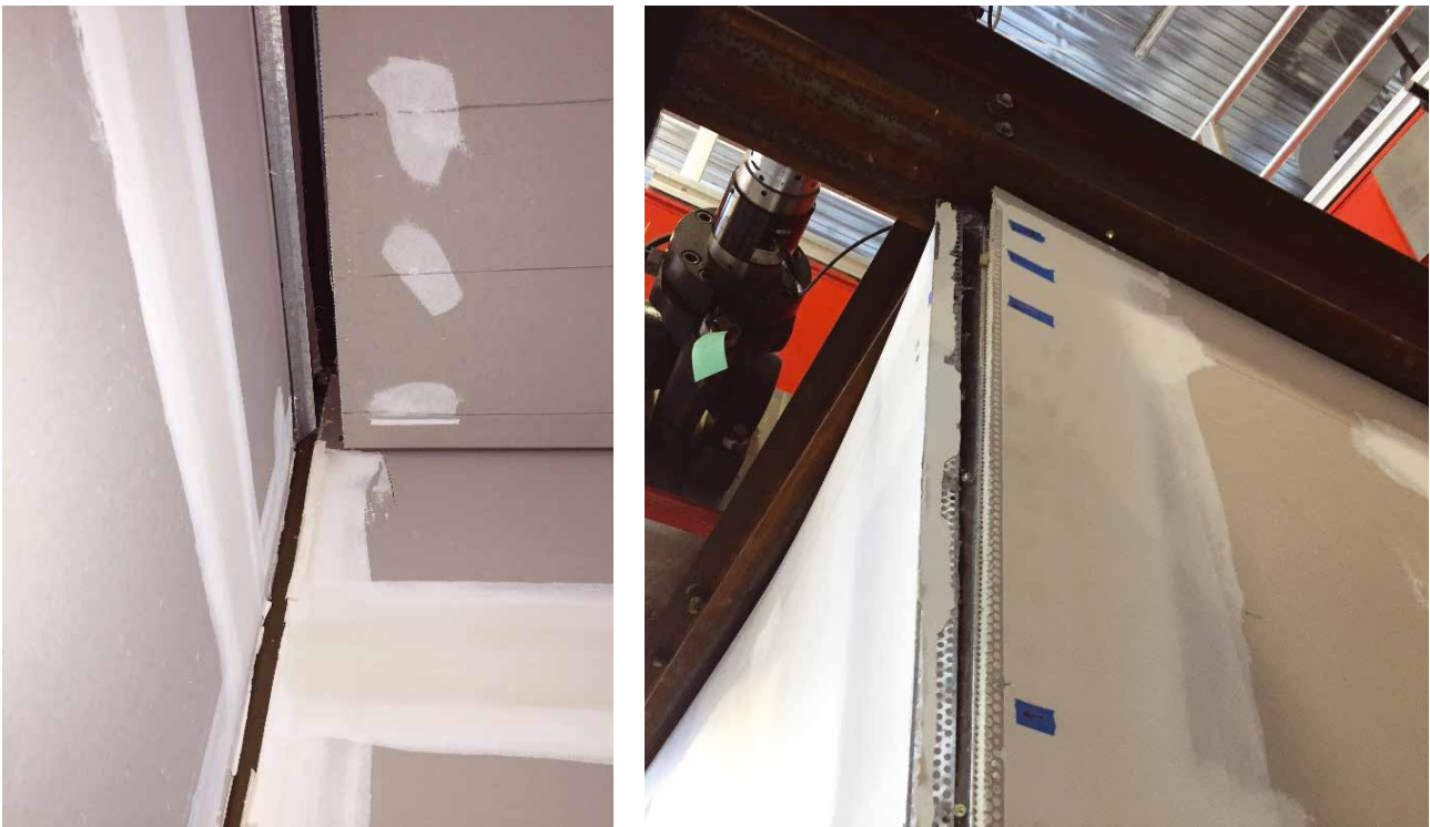
■ PHOTOS 6 & 7 – 1.5% DRIFT (40.5MM) INTERNAL CORNER, CEILING JUNCTION AND EXTERNAL CORNER
